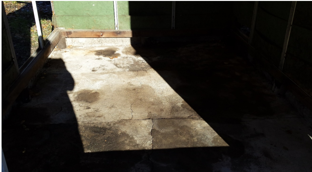
Shed with staining.
